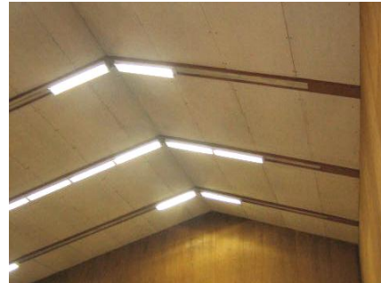
T-5 fixtures save energy while greatly improving light levels in large spaces.
