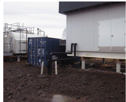
Completed heat recovery lines exiting the Power Plant
