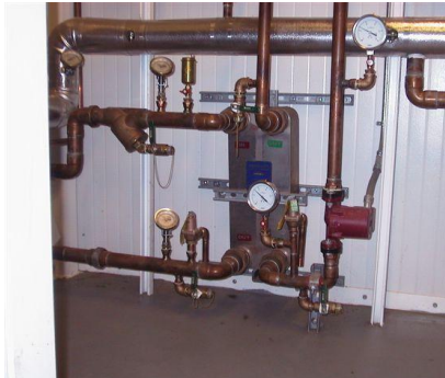
Plumbed and operational heat exchanger harvests hot water from generators and transfers to boiler supply lines
