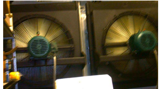
Fans in the power plant were regularly dumping true "waste heat"
